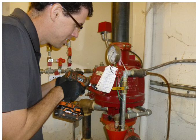
Educating stakeholders regarding the purpose of the inspections and tests mandated by NFPA 25 is an ongoing challenge.
