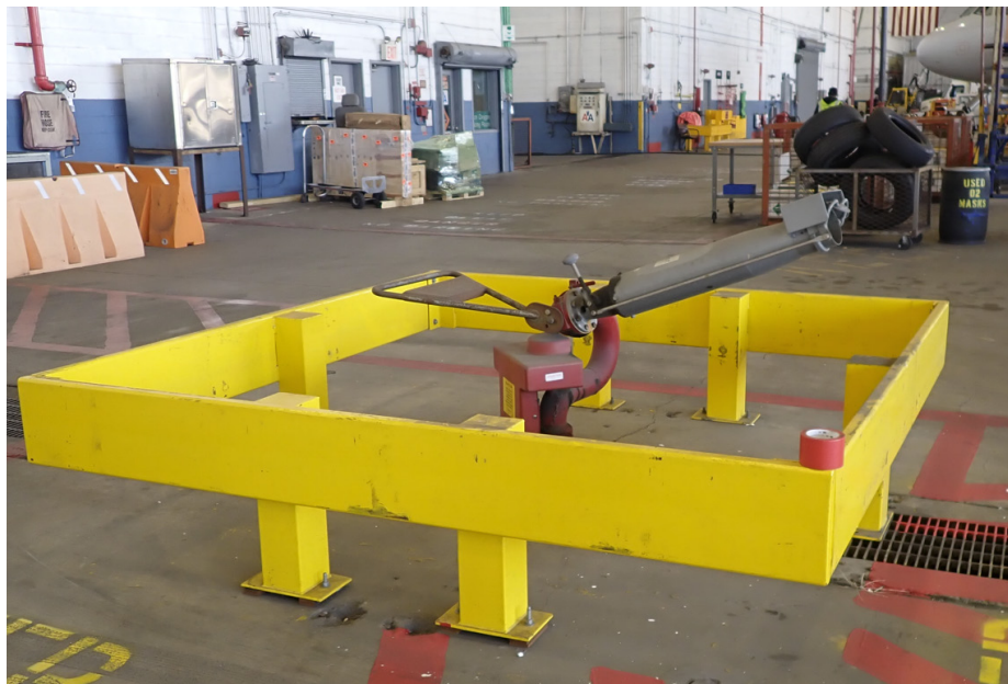
Figure 2. Ground-level foam monitor.
