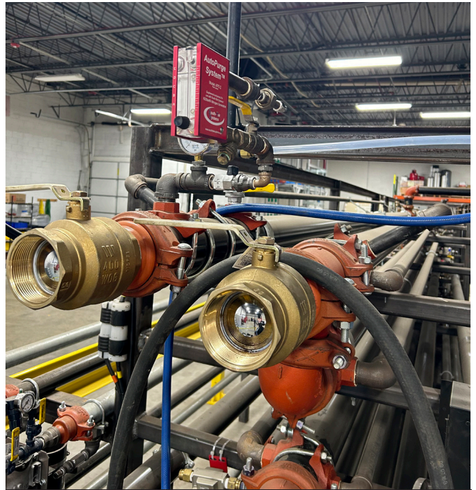
Figure 7. Continuous purge valve for Test 3.
